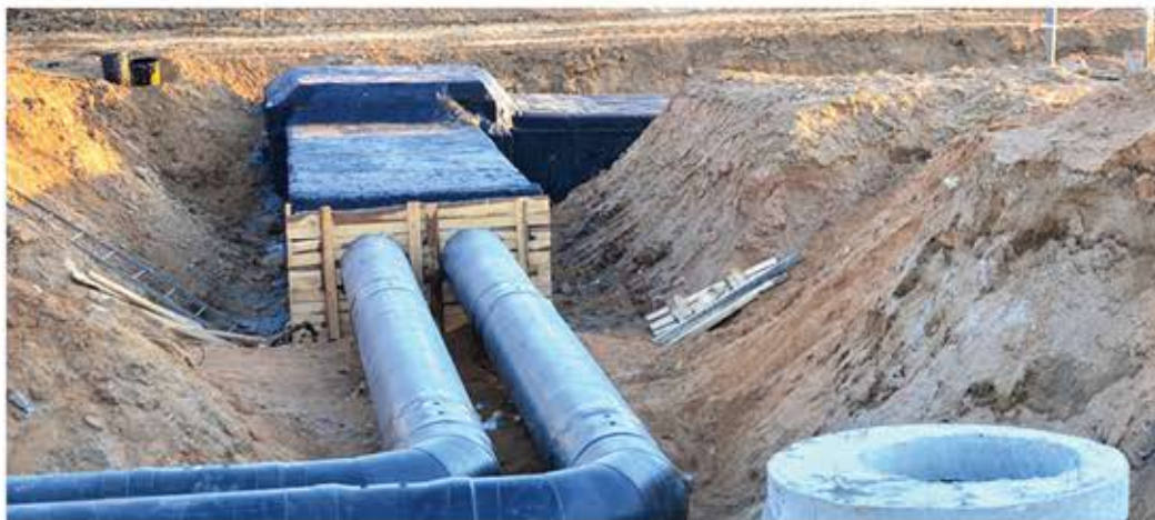
STRONG UNDERGROUND DRAINAGE SYSTEM
